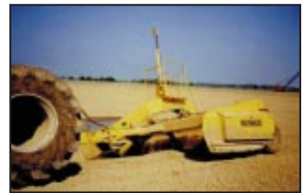
Figure 2. A small dirt pan (dirt bucket) is used for finishing work in rebuilding levees.
